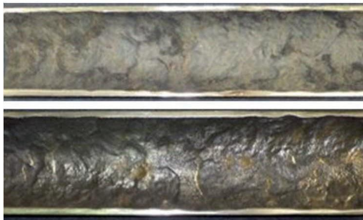
FIGURE 2. Pipes of the installation affected by corrosion under the tank
