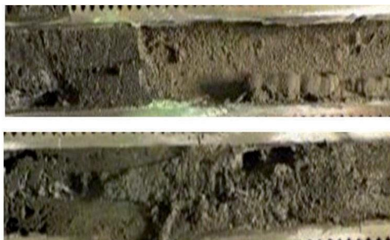
FIGURE 3. Heat exchanger tubes blocked due to high deposit build-up
